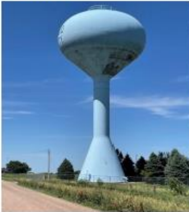
Figure 5. 750,000-gallon elevated water storage reservoir
